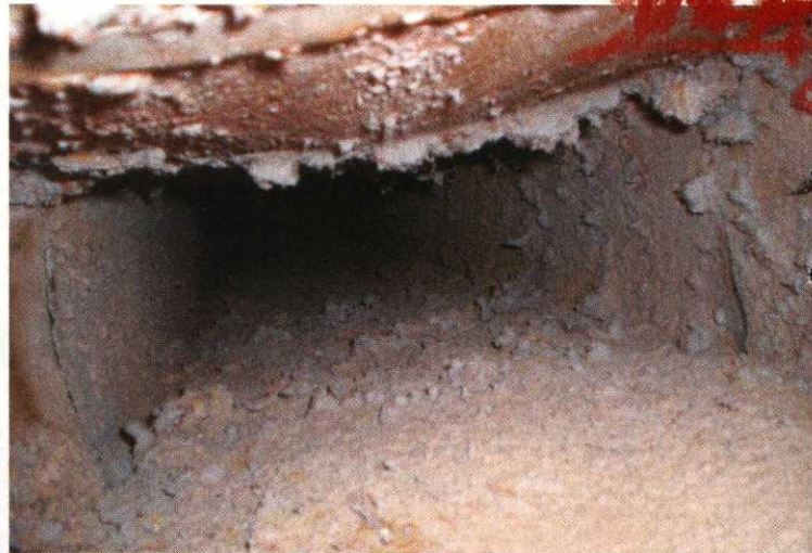
An example of a dirty, low-wall return-air duct in need of cleaning.
