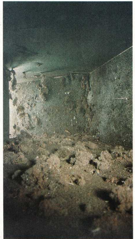
The amount of debris in ductwork can surprise home and business owners.
