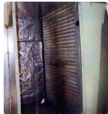
Inner view of a dirty air and heating unit that needs cleaning.
